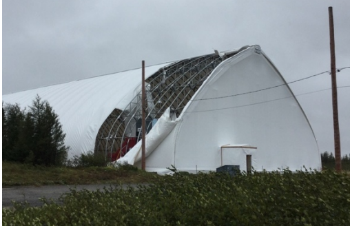
Figure 11: Roof of the Chevery Arena Ripped off by Extreme Wind Gusts
